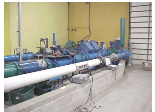
Ultrasonic Meter Test Line
